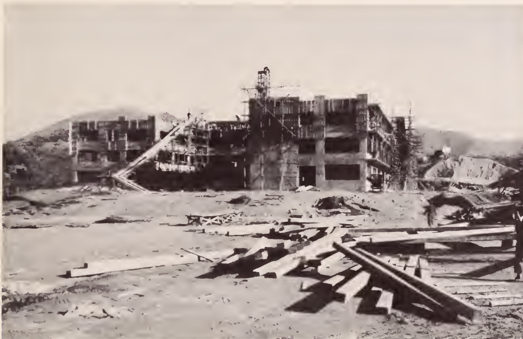
The Eighth U.S. Army Memorial Chest Hospital is already half built. The largest AFAK project will be completed by next summer. (U.S. Army Photo)
